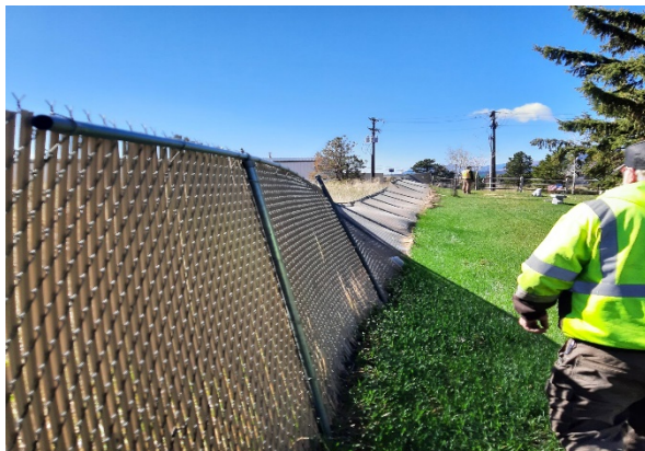
Pre-Existing – Damaged Fence (removed)
