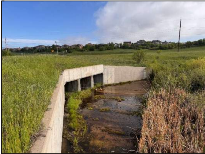
Photo 14: J05-struct01. Jackson Creek at Leather Chaps Drive. Downstream end choked with cattails and sediment. Upstream pond serves as regional detention facility, poorly maintained.
