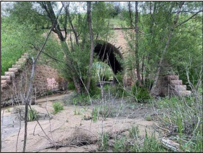
Photo 9: D10-struct01. Dirty Woman Creek at New Santa Fe Regional Trail. Large bridge/tunnel structure, filled with sediment. Downstream culvert clogged, leading to overtopping.
