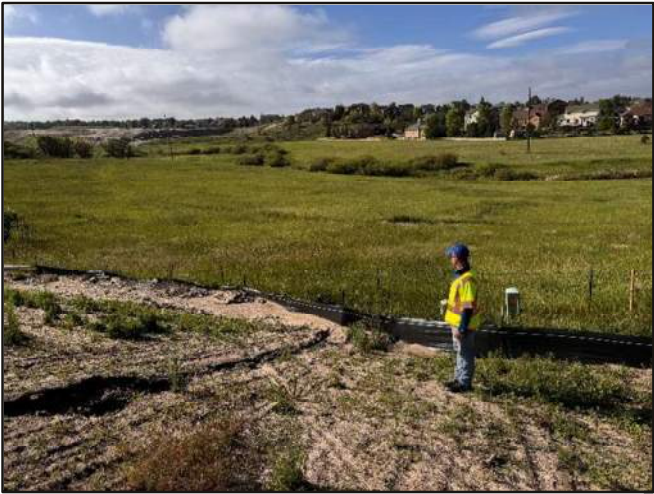
Photo 18: Jackson Creek development north-east side (upstream end) of Leather Chaps Drive. Poor erosion control measures.
