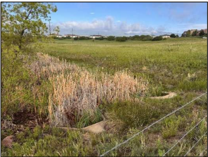
Photo 17: J05-struct02. Jackson Creek at Leather Chaps Drive. Outfall clogged with cattails.
