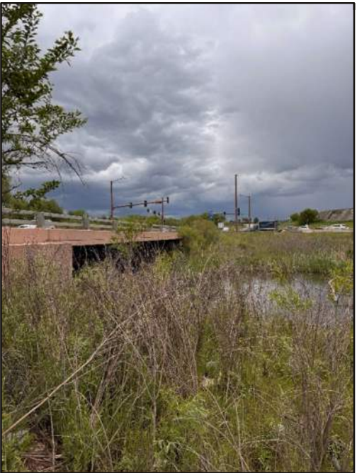
Photo 10: D17-struct01. Dirty Woman Creek at W Highway 105. Standing water and possible blockage. Large ponding issues seemingly due to overgrowth.
