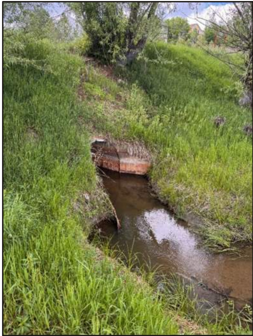
Photo 6: D02-struct01. Dirty Woman Creek at Knollwood Drive looking north (upstream side). Signs of deterioration, flow unobstructed.
