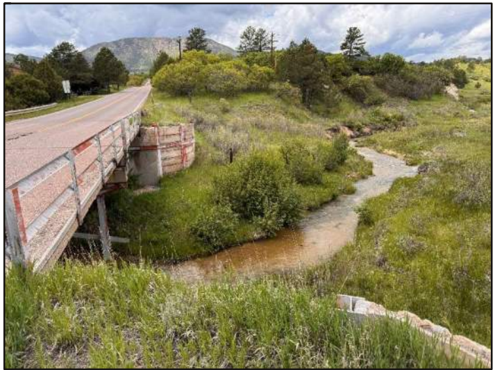
Photo 21: Monument Creek looking north, erosion upstream of Mt. Herman Road bridge.
