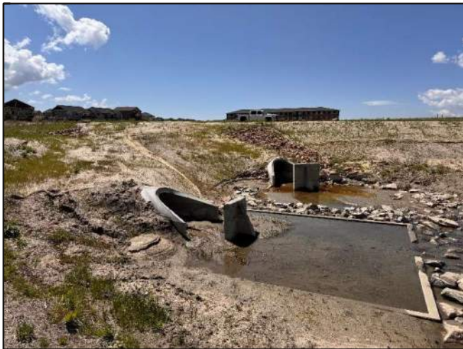
Photo 33: North Teachout basin upstream of Jackson Creek Parkway. East side outfalls looking SE. Poor erosion control measures. Erosion and sedimentation visible.
