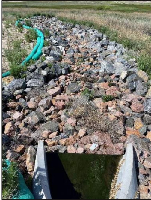
Photo 32: T05A-struct03. At intersection of Higby Road and Bowstring Road. Riprap insufficient for expected flows, ends at PL, channel incised.
