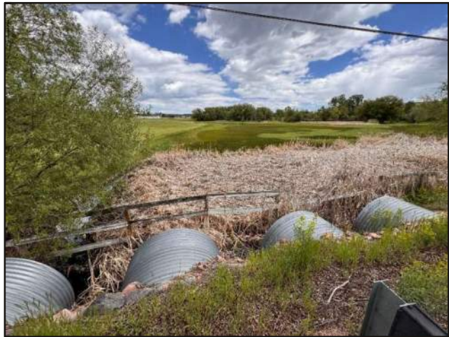
Photo 1: C02-struct01. Crystal Creek at N Monument Lake Road. Upstream has wide flood area with vegetation clogging.
