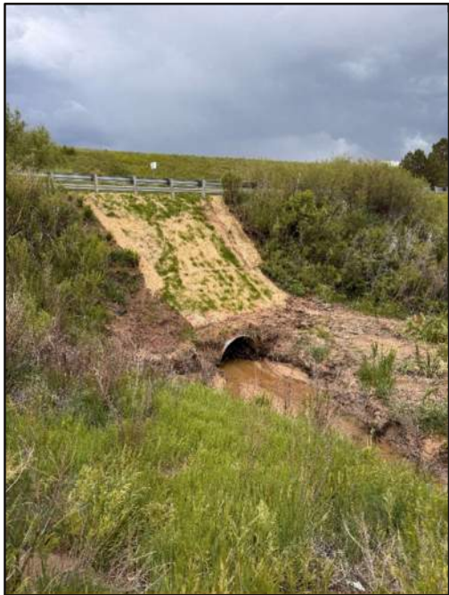
Photo 8: D04-struct01. Dirty Woman Creek at Old Denver Road. Completely clogged and deformed, erosion matting suggests possible overtopping. No longer functional.
