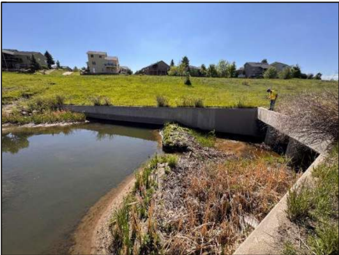
Photo 13: J03-struct01. Jackson Creek at Jackson Creek Parkway. Sediment buildup and upstream failures. Series of ponds/dams along Jackson Creek with flatland overflows with 10+ ft erosion incisions.
