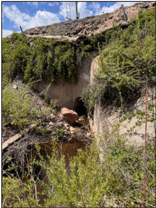
Photo 24: T01-struct01. Teachout Creek at Union Pacific Railroad (south). Sediment buildup, overgrowth.
