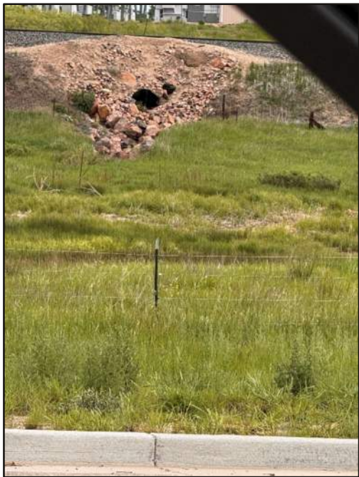
Photo 27: T02C-struct01. Teachout at Union Pacific Railroad, west of electrical substation looking west. Washed out culvert.
