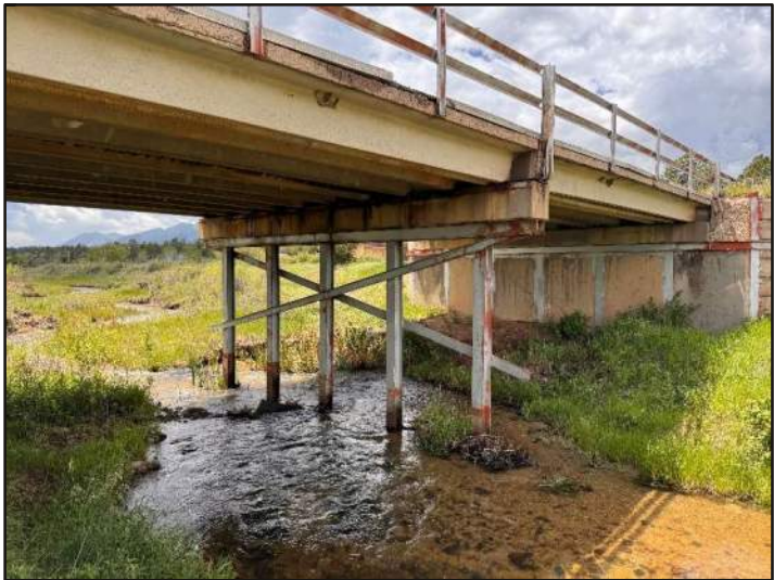
Photo 20: M14-struct01. Mt. Herman Road bridge over Monument Creek looking SW. Roadway Deteriorating, steel beams in creek causing erosion, abutments deteriorating, erosion both upstream and downstream.
