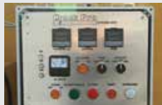
Digital Control Center with Protective Steel Cover
